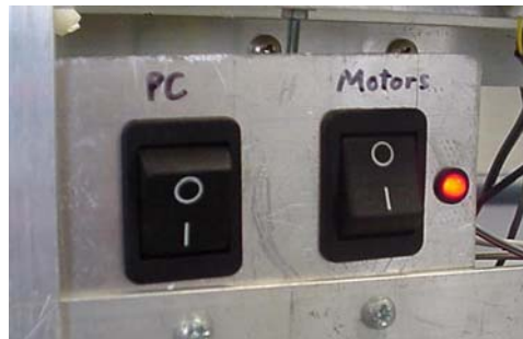
Figure 2.4: Power Switch Panel
